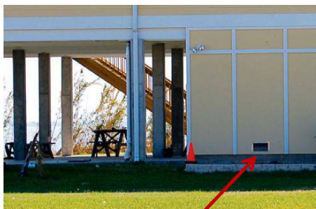
Flood opening in a below-BFE enclosure wall.
