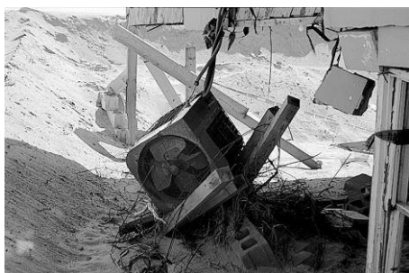
Electric heat pump dislocated from its shattered wooden stand by velocity flow in a coastal area
