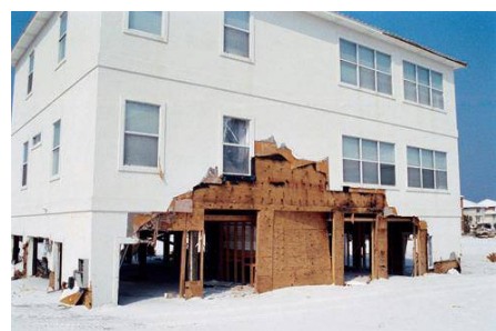
Building siding extended down and over the breakaway wall. Lack of a clean separation allowed damage to spread upward as the breakaway wall failed.
