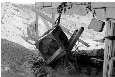
Electric heat pump dislocated from its shattered wooden stand by velocity flow in a coastal area
