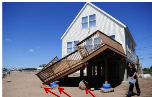
These footings appeared to have been subjected to scour or erosion from wave action
