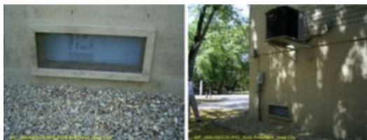
A house where flood openings have been covered by insulation and drywall
