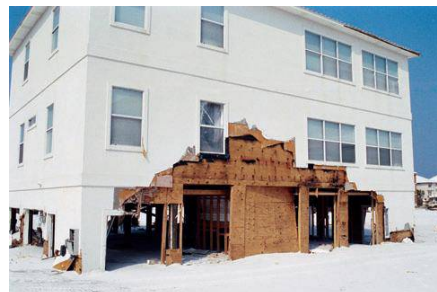
Building siding extended down and over the breakaway wall. Lack of a clean separation allowed damage to spread upward as the breakaway wall failed.
